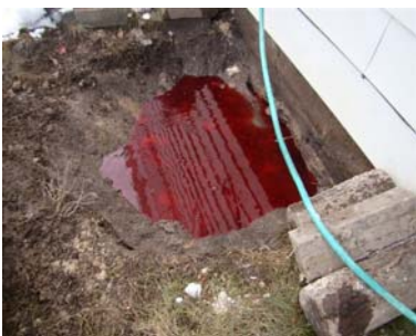
A hole full of fuel was discovered adjacent to the storage tank.
