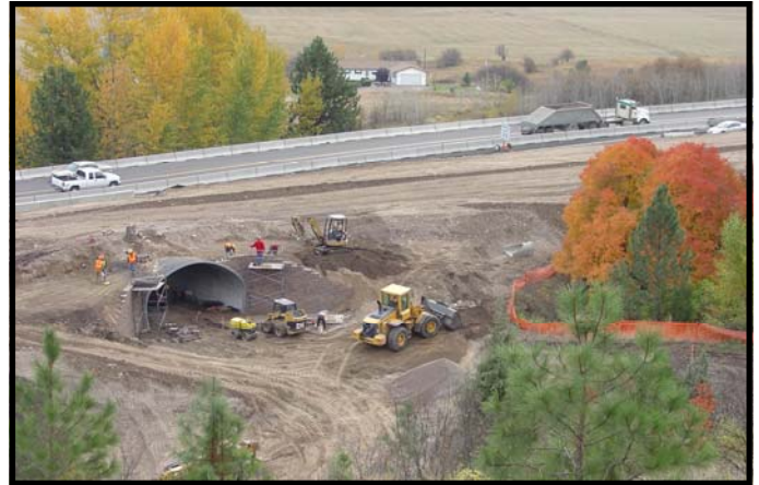
Highway 93 wildlife crossings at bottom of Polson Hill
